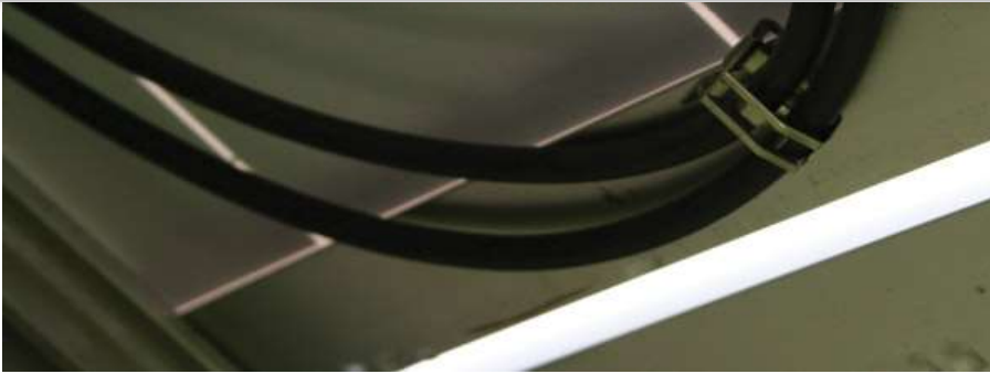
Photo 1. Conductors that are properly supported to the module frames are less likely to cause long-term problems. Various products are now available that are designed to clip to the module frame and hold PV conductors in place.
